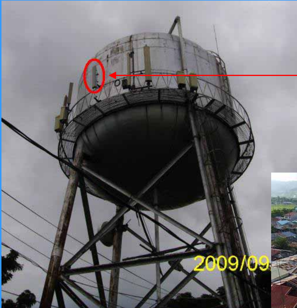
5-watt AP with 120-degree sector antenna on water tower
